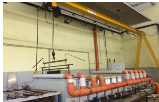
Figure 4 Production line of surface treatment
