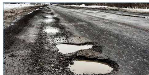
Figure 2 The potholes on the road surface (tirereview.com, 2021)
