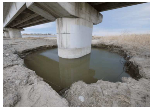
Figure 1 the pier scours at the eastern Yuriage Bridge Kayen
