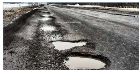
Figure 2 The potholes on the road surface (tirereview.com, 2021)
